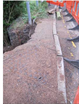
Gabion baskets installed before June 2009, disjointed kerbing, sloping metal posts of the safety barrier.
